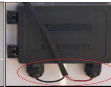
Fig.4. Too Short Wire
