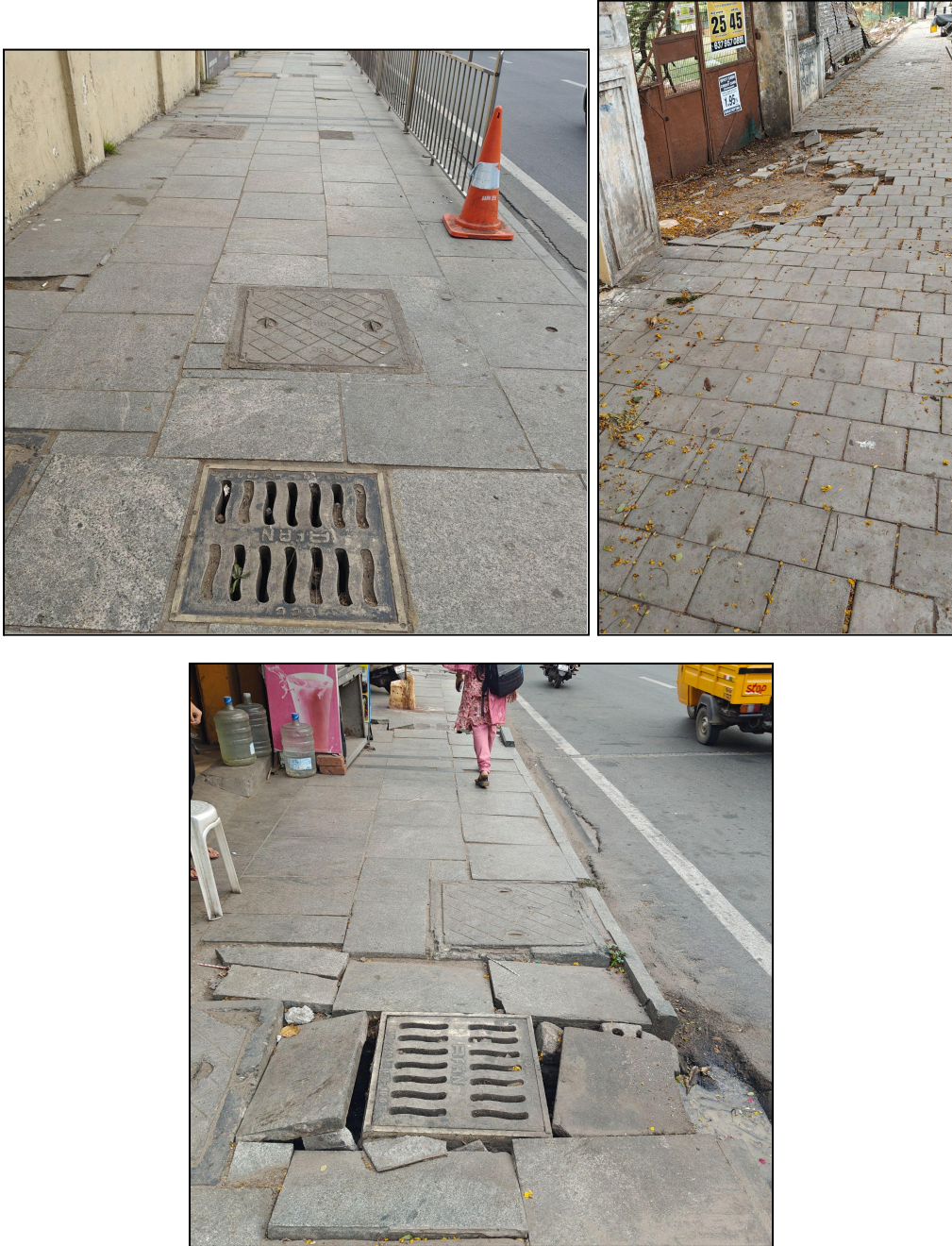
Uneven footpaths with poor maintenance on the Jane's Walk route CAG
