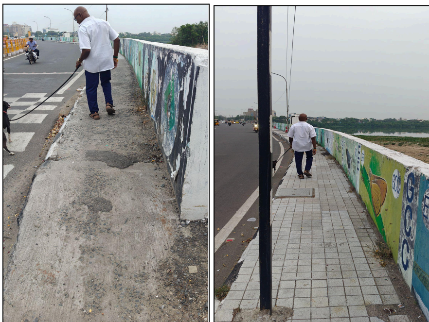
Pedestrian using the footpath on the Adyar Bridge (Thiru-Vi-K-Bridge) and not finding enough space for his pet on the footpath| CAG
