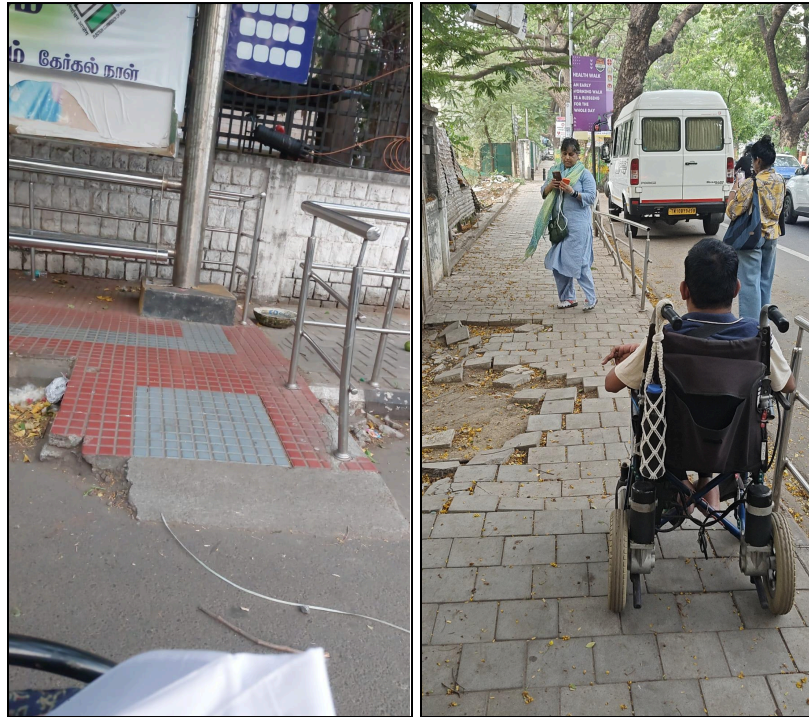
Broken ramps and footpaths acting as hindrances to accessibility on the Jane's Walk route
