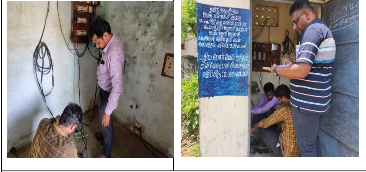
Photo : Power quality measurements of OHT pumps being carried out by CAG team in Kadambathur Panchayat
